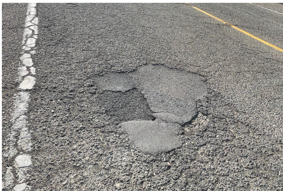
Photo 2: Section 2 Raveling, Alligator Cracks and Failed Patching
