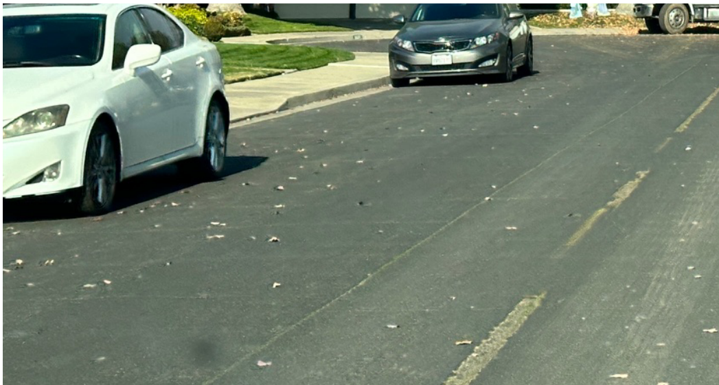
Photo 1: Section 1 Moderate Longitudinal Cracking
